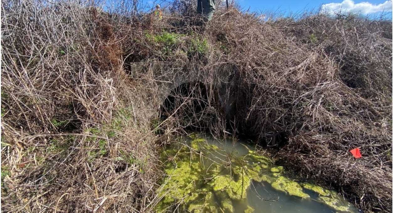
7. Facing northeast at downstream outlet of culvert on south side of rail.
